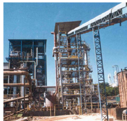
REACTOR TOWER WITH BAGASSE FEEDING SYSTEM
